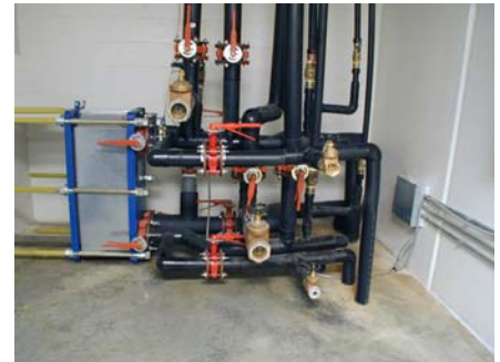
Stainless Steel Plate and Frame Heat Exchanger connected to closed loop system.
