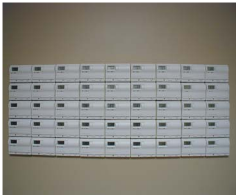
Individual classroom temperature controls located in one central location.
